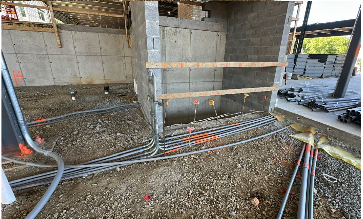
Underground Electrical Conduits in the Multipurpose Wing.
